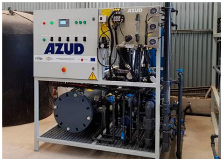
Pilot plant for the study of regeneration of treated wastewater
